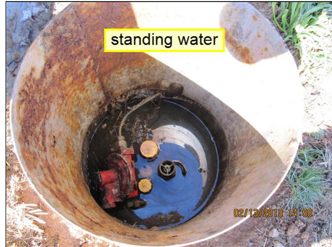
6.4 Item 2(Picture) propane tank valves
